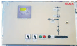
SEPAM (SCHNEIDER ELECTRIC)
