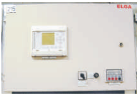
MiCOM (SCHNEIDER ELECTRIC)
